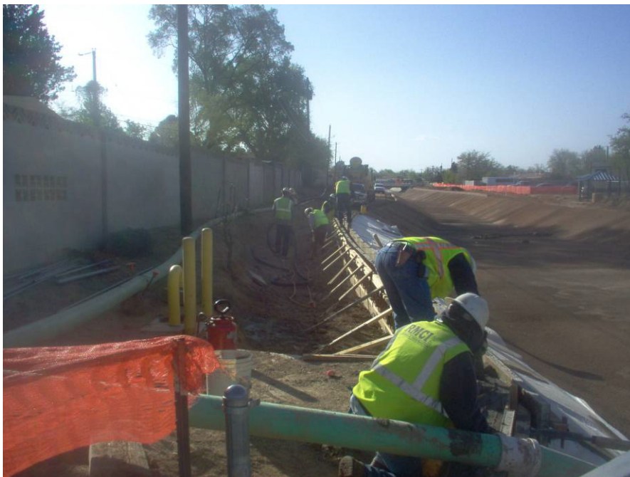
RMCI crews finishing concrete on sill wall north side of the channel east side of the San Pedro Bridge.
